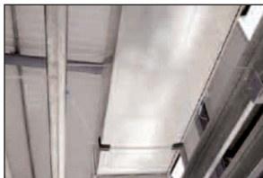
Square Air Ducts
